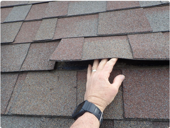
Stonebriar field photo: shingle tabs lifted by hand during a roof inspection. Wind and hail damage is often hidden from the ground; a qualified roof evaluation documents it.
