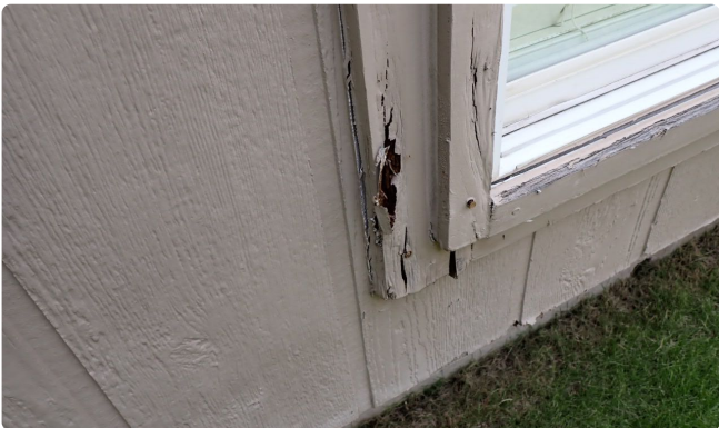
Stonebriar field photo: deteriorated trim where siding meets soil and chronic splash.
