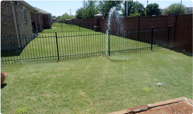
Stonebriar field photo: spray zones should water plants and turf, not walls, windows, or equipment.
