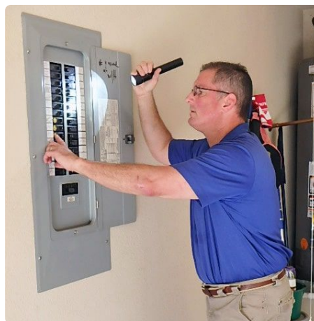
A professional inspector examining an electrical panel. Homeowners should observe a closed panel from a safe position and never remove its cover.
