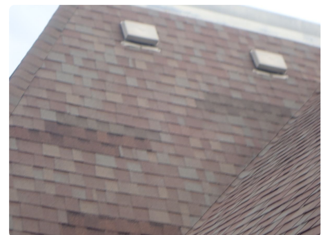
Stonebriar field photo: roof vents and penetrations are common leak points; note them in your photo route.
