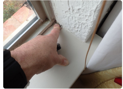
Stonebriar field photo: checking a gap at a window sill. Window leaks may start at the window, the wall, or the flashing; record when water appears before choosing a repair.
