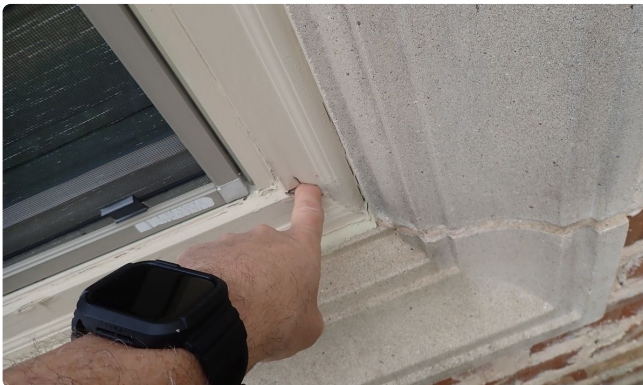
Stonebriar field photo: an open joint at a window sill and masonry trim.
