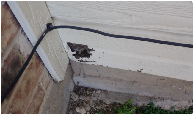
Stonebriar field photo: damaged lower siding and trim at a wall corner. Clearance and drainage help prevent this pattern.
