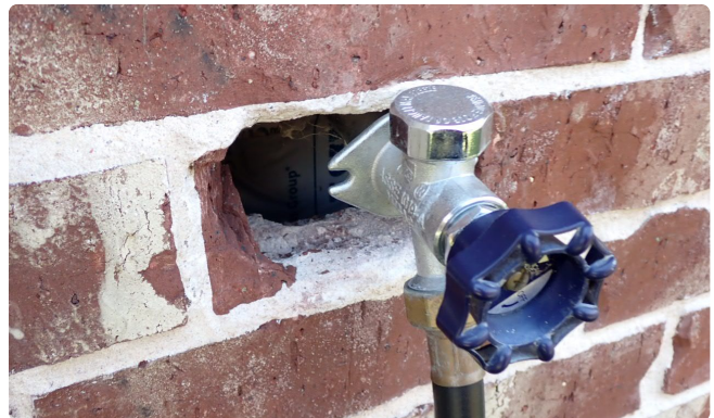
Stonebriar field photo: an exterior faucet penetration with missing mortar around the opening.
